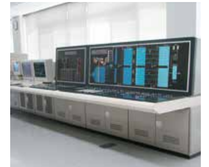
Sewage activity monitoring room
