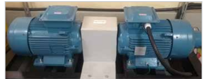
Motor loading facility – 22kW
